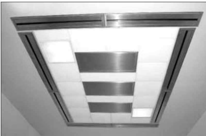
Photo shows standard 12 x 8 Steri-System module installed in the Nailor Air Distribution laboratory.
